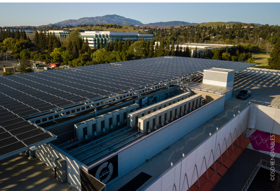
DSD's 1.28 MW solar, 1.3 MWh storage installation at Bishop Ranch business park, San Ramon, Calif.
